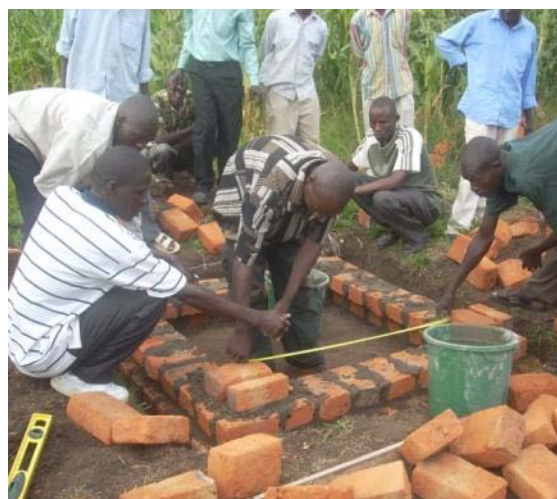
Picture 21: Constructing a corbelled brick foundation (Notice the offset of the upper course of bricks)
