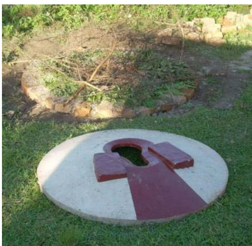
Picture 24: Dome slab ready to be placed on foundation (in background covered with branches to cover pit)
