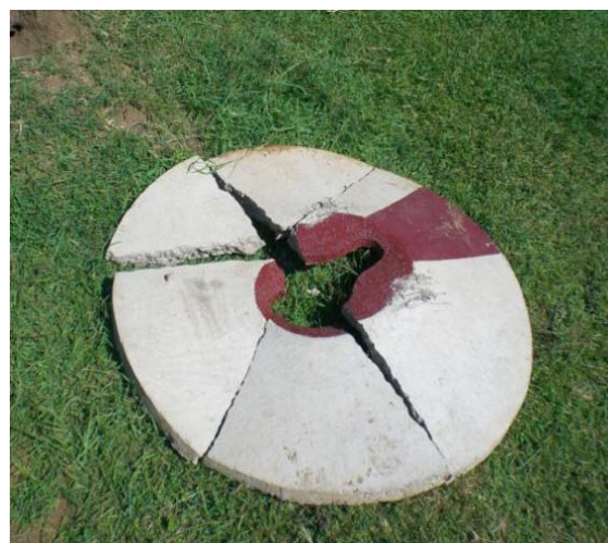
Picture 16: Cracked dome slab that was dropped
