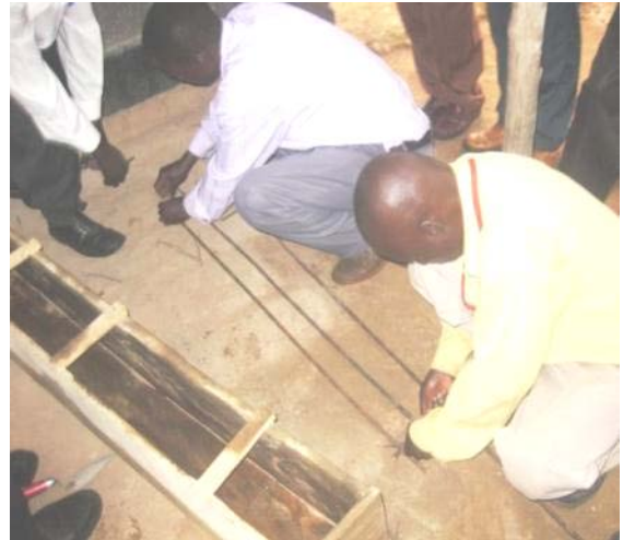
Picture 11: Preparing iron bars for the concrete beam for a double stance latrine
