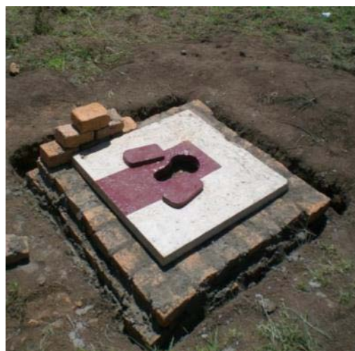
Picture 25: Completed Square Reinforce concrete slab with foot rests and epoxy paint
