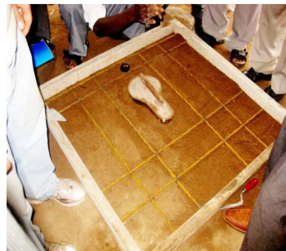
Picture 9: Finished mould for square reinforced concrete slab, with reinforcing bars and drop hole mould
