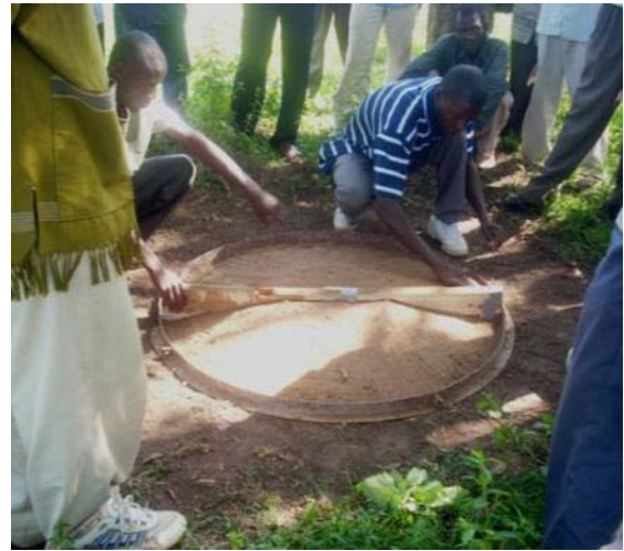
Picture 8a: Completed sand pile, prior to placing the drop hole mould
